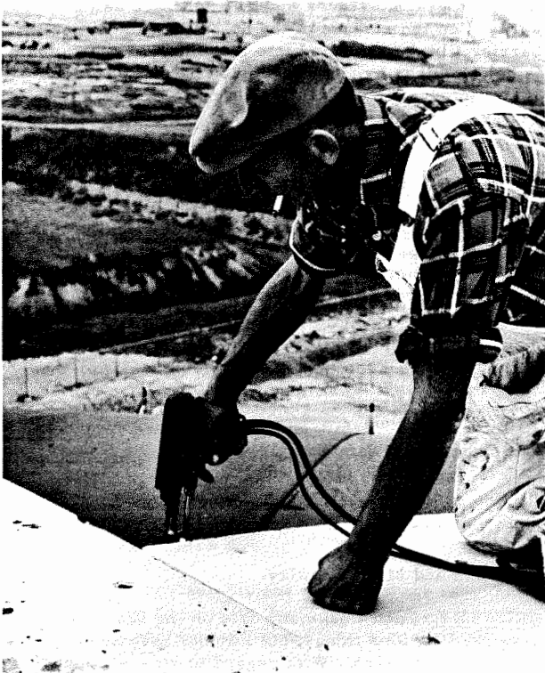
Figure 4. Method of attaching stud welds to the roof with a stud gun.
